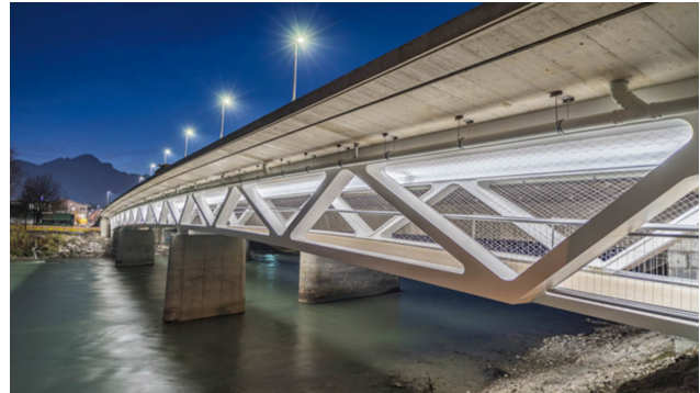
Fig. 4: The object of interest is the part of the Grenobler Bridge used for public transport, foot- and bike traffic.
